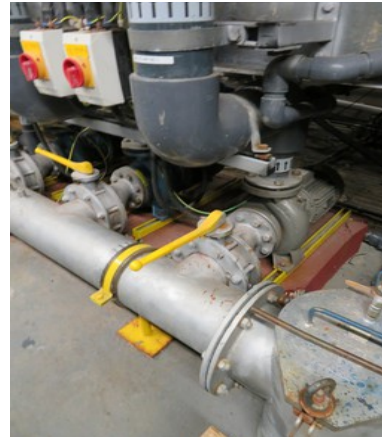
Indoor Pools Pump and manifold
